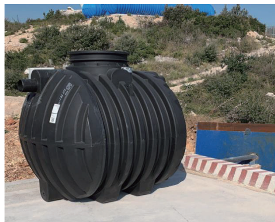
Fig. 40 Oil water separator set in concrete tank car parking area
