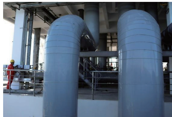
Fig. 64 Oil pipeline of oil terminal of Mombasa Port
